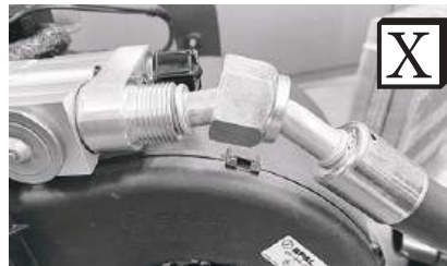
Improperly Seated O-ring Land
